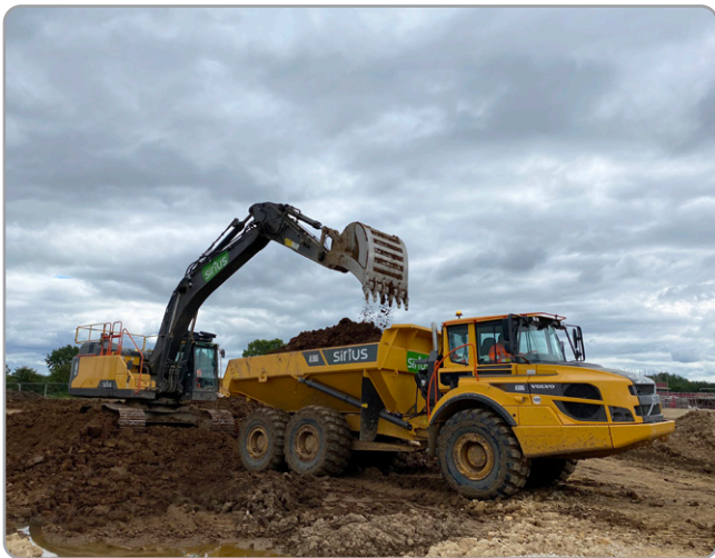
Sirius has a fleet of the most up-to-date, fuel-efficient machines equipped with GPS for the most efficient and accurate works
