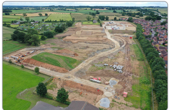
View of the site looking south during the roads and sewers installation phase
