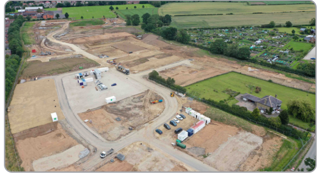
View of the site looking north during the Sirius Civils team roads and sewers installation phase
