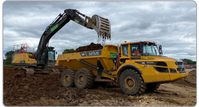
Sirius has a fleet of the most up-to-date, fuel-efficient machines equipped with GPS for the most efficient and accurate works
