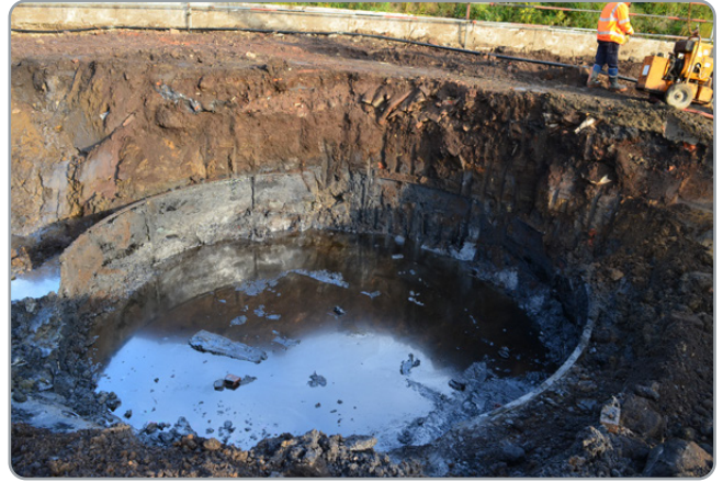
Old tar and fuel tanks had been left buried underground
