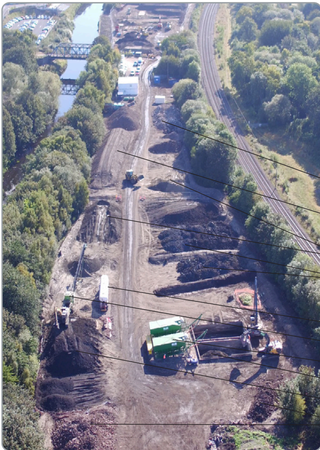
Sirius site specific treatment area
