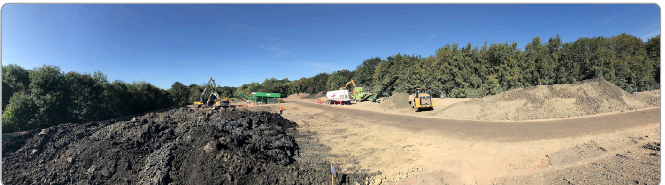
Dark, tar contaminated material on the left before treatment
