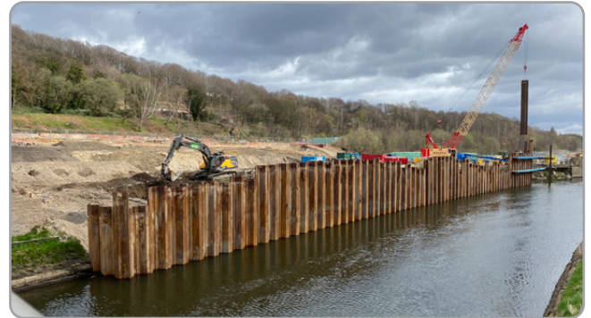
Installation of a temporary sheet pile wall in the river creating a dry working area to carry out earthworks and river wall construction
