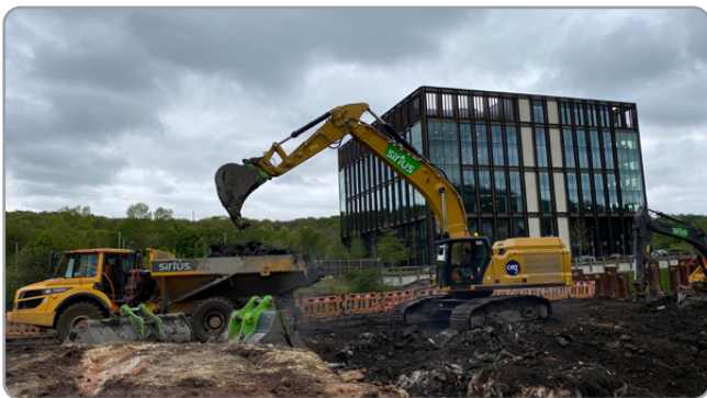
Earthworks turnover with removal of contaminated materials and obstructions as they are identified
