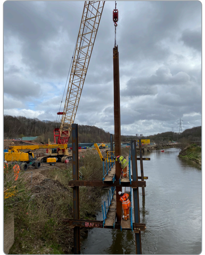
The initial steel frame construction to assist in building the temporary sheet pile wall in the river
