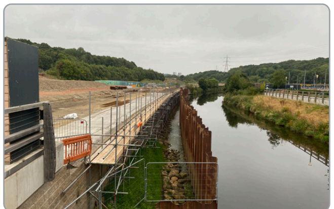
Construction of reinforced soil steps and Allan block wall, with rip rap (coarse rocks) placed at the foot of wall to mitigate river erosion
