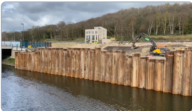
Temporary sheet pile wall completed in the river enabling earthworks and the construction of a new river wall behind the sheet piles
