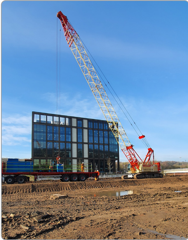
The crane unloads materials for the construction of the temporary sheet pile wall
