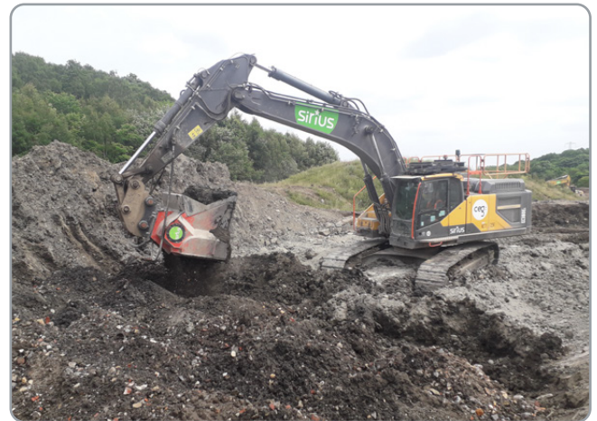
Excavator fitted with stabilisation bucket mixing stabilisation/solidification binder into hydrocarbon contaminated soils
