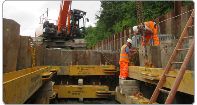
Positioning bracing inside sheet piles to enable the installation of large below ground interceptors
