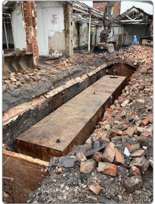
Heating oil tank inside one of the arches in Building 2 – tank contains heavy heating oil. To be cleansed/degassed and removed
