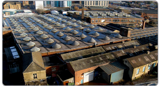
View of the Temple Works roof with its 66 equidistant glass conical skylights and the demolition site to the right
