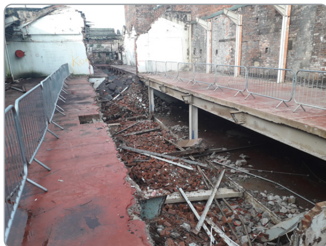
Break in slab and arches within Buildings 3 & 2 respectively
