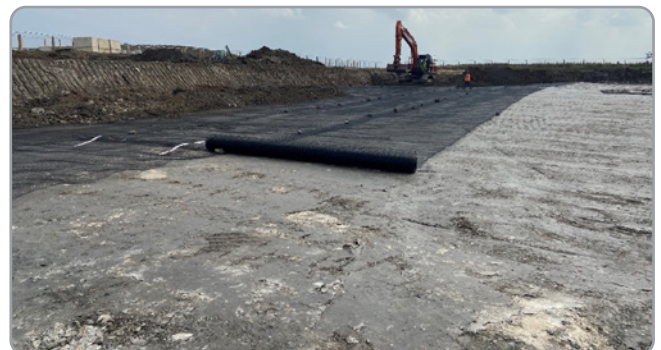
Geogrid placed with 0.5m minimum overlap on base of excavation prior to placement of engineered fill
