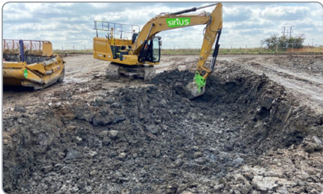
Excavation works expose 'colliery spoil' beneath 'capping clay'. Material relocated for quarantine and tested for any residual contamination
