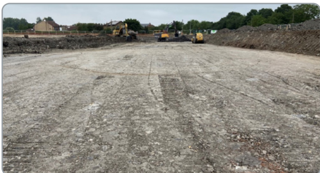
Base of excavation civilised and proof rolled prior to placement of geogrid
