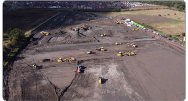
After excavation of soils and installation of geogrid, the placement of engineered fill and compaction is carried out
