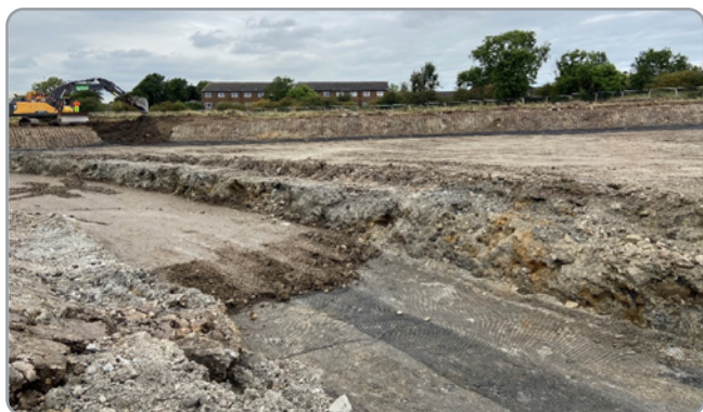
Placement of engineered fill in 0.2m thick layers over geogrid within road box cut
