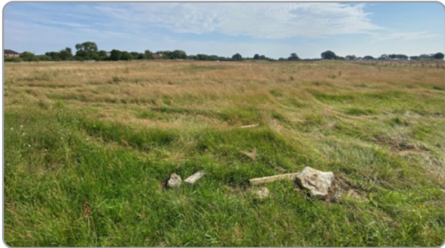
View east across KO1 to KO3 prior to remedial and preparatory earthworks
