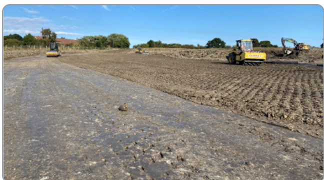
Compaction of engineered fill by pad foot and smooth drum rollers working in tandem
